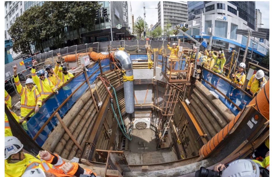
Micro boring tunnel machine breaks through at Victoria St East after laying a new wastewater pipe under Queen St
