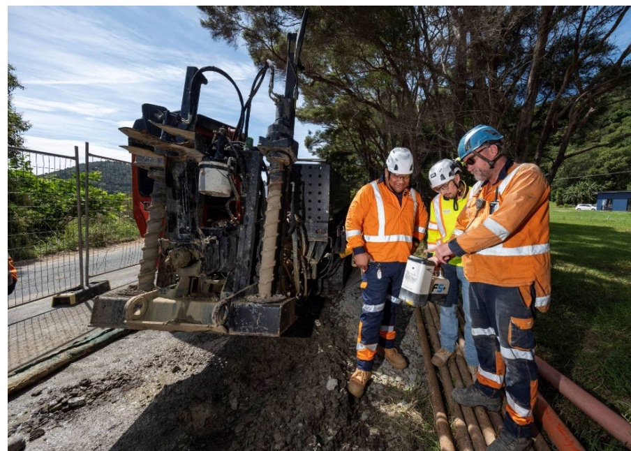
Crews work to install a 4.5km wastewater main that will transfer wastewater from Waiwera to Hatfields Beach pump station
