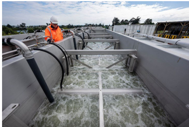
Activated sludge 'bugs' settle into their new environment at Clarks Beach Wastewater Treatment Plant.
