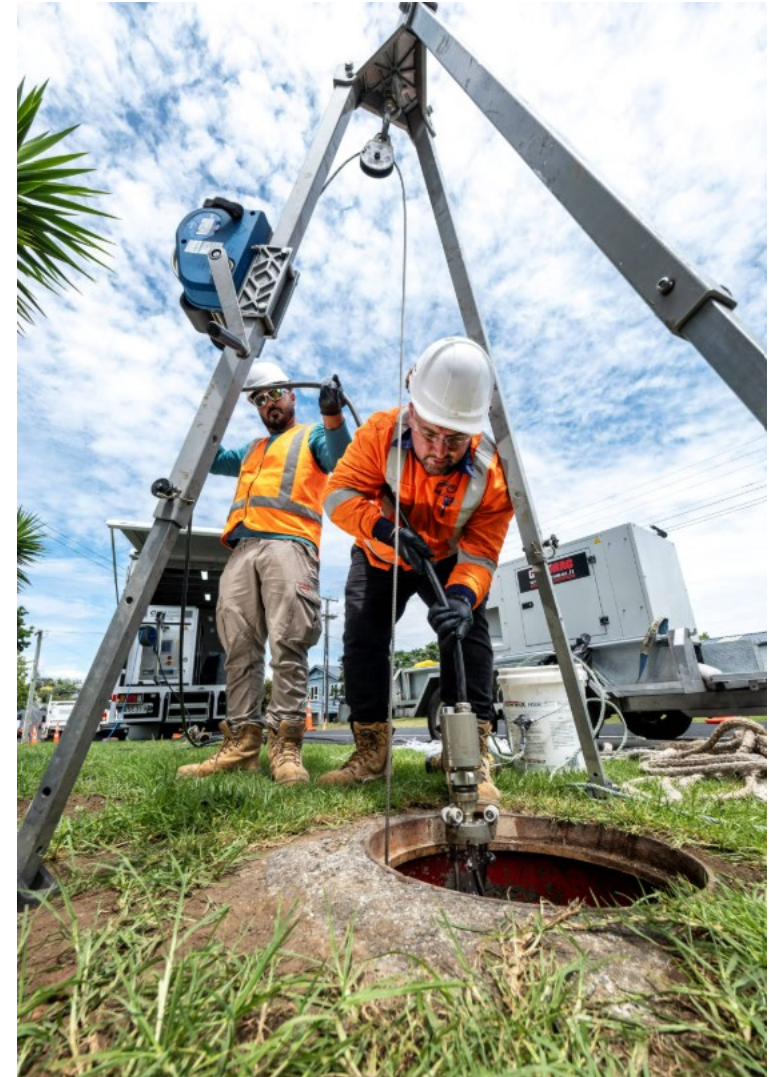
A small CCTV rover is lowered into the manhole to assess the condition of pipes in Beachlands and Maraetai before relining is carried out.
