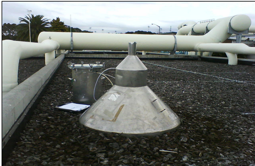
Figure 14: Sampling Primary Sedimentation Tank biofilter (zone 1)
