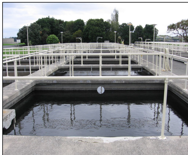
Figure 10: CAS Tank at Rosedale WWTP.
