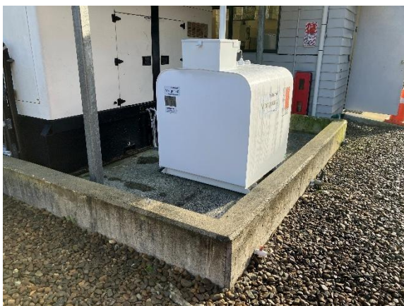
A: Diesel storage tank in concrete bund
